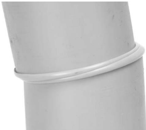
“high-low” pipe alignment. Visually mitered joint.
